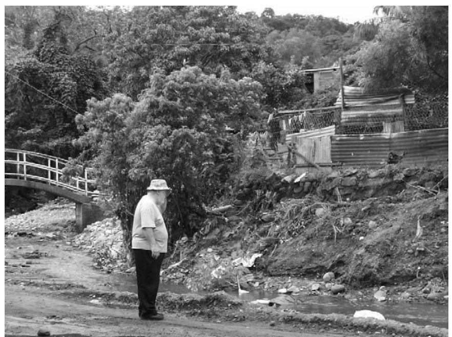
Ross Menard surveys flood damage at a minor tributary of the main river in Matagalpa. During the rains, water reached 20 feet deep at this point.
